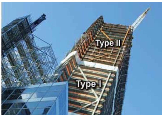
Non-combustible building elements are atop fire-resistant elements in this high-rise tower under construction.
