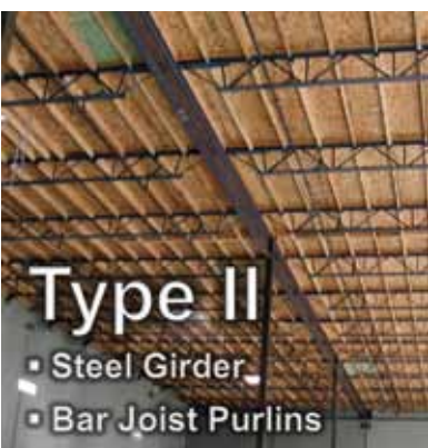
Type II hybrid building featuring unprotected roof structure and wood roof deck.
